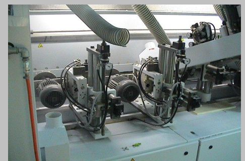
Disc sanders installed on the edge sander.
